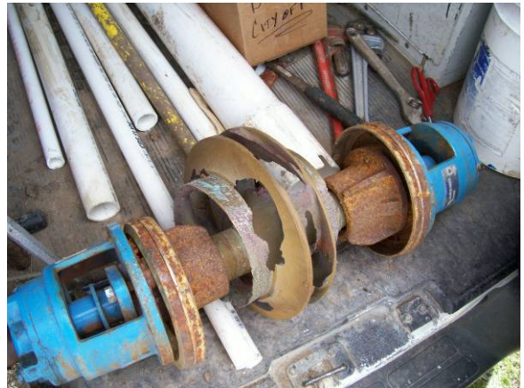
Impeller damage after 18 months of operation with improper pump/motor combination.
