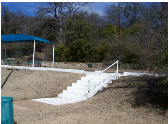
Stairs have only one hand rail, which is broken. There is a trip hazard at the top of the stairs.
