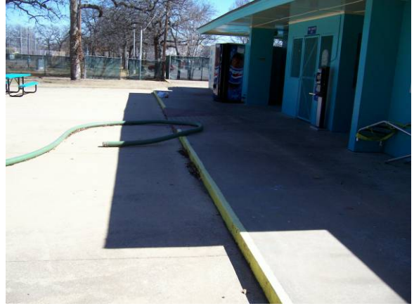
Step in front of bathhouse without handrails.
