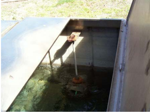
Severe corrosion on valve handle.
