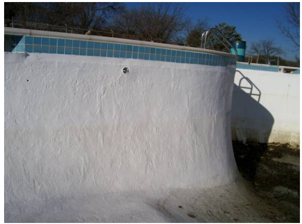
Rough condition of pool deck.
