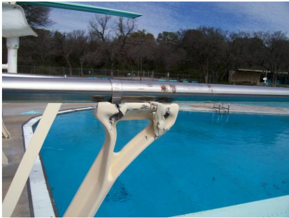
Diving stand railing brackets are broken. (Reported to have been repaired in annual maintenance by staff for 2007 season.)
