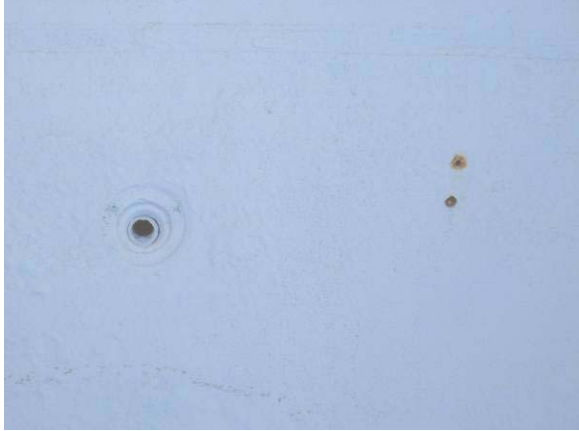
Wall inlet is missing eyeball fixture. Small holes, purpose unknown, are causing corrosion staining on pool shell.
