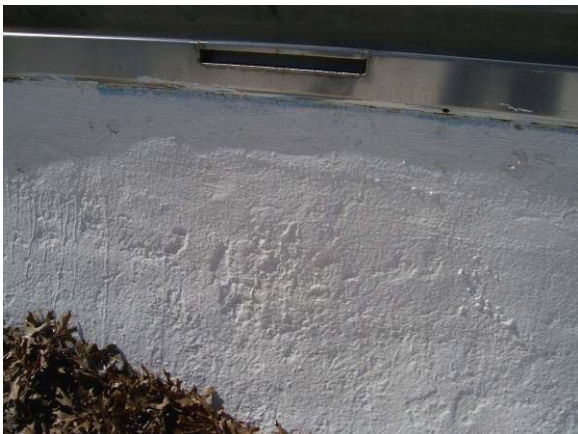
Rough condition of pool shell
