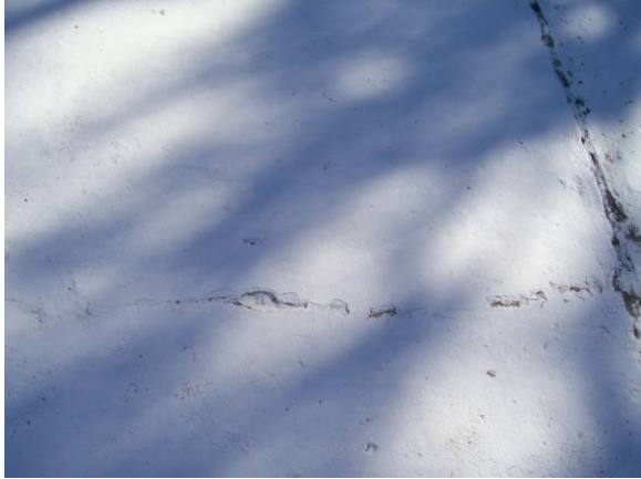
Large cracks and rough surface of pool shell.
