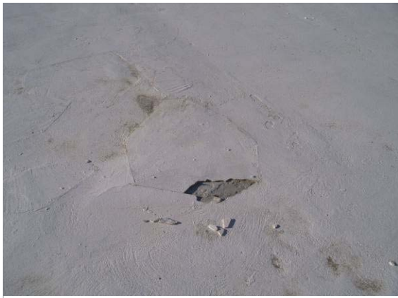
Patching in deck is failing.
