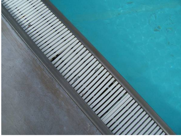
PVC grating is in poor condition.
