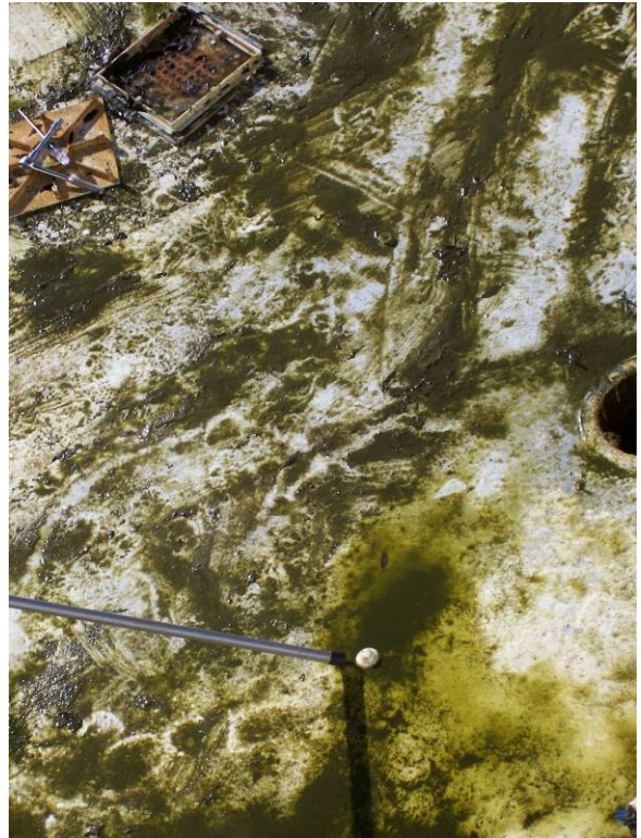
Objects protruding through pool shell believed to be formerly used as drains.
