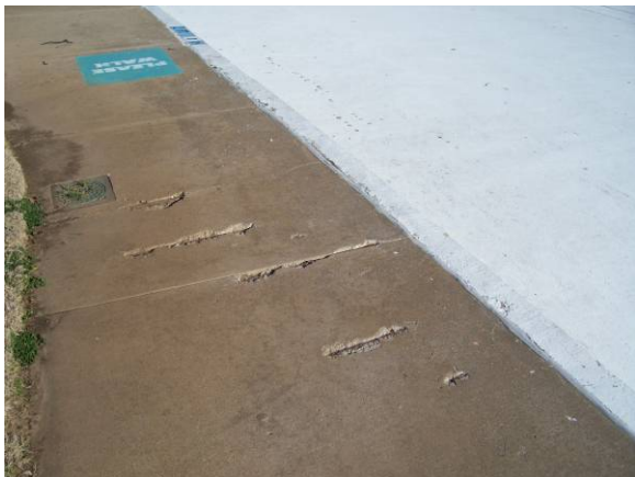
Exposed rebar in pool deck.
