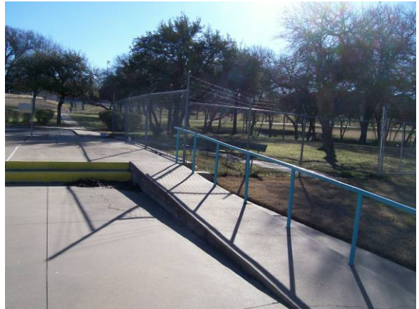
Sidewalk ramp with only one handrail.
