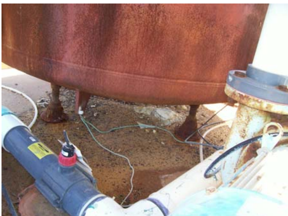
Severe corrosion of filter tank legs.
