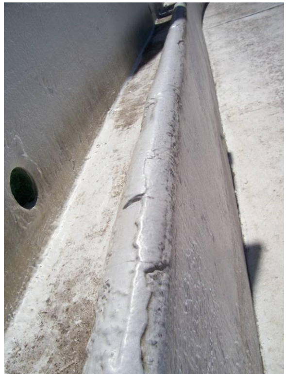
Spalling concrete along gutter lip.
