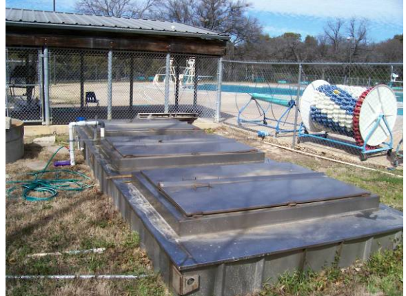
Stainless steel vacuum sand filter vault.
