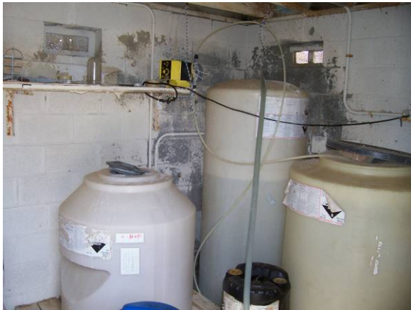
Single walled chlorine and acid containers stored in the same room.
