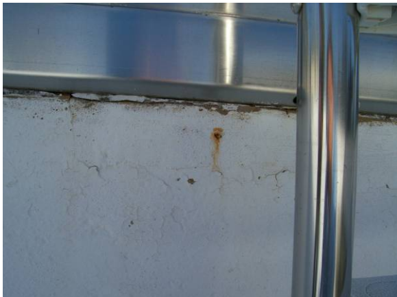
Corrosion believed to be caused by rebar positioned near the pool shell surface, poor joint between stainless steel gutter and concrete pool shell.
