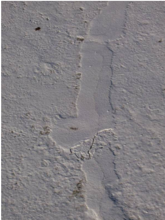
Pool crack repairs are failing.
