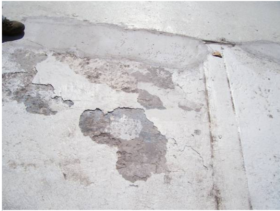
Multiple patches and rough condition of pool shell
