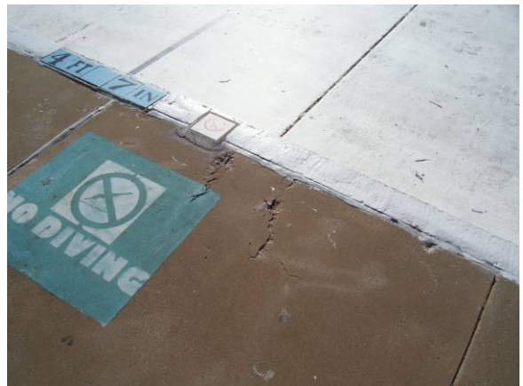
Poor condition of deck and coping.
