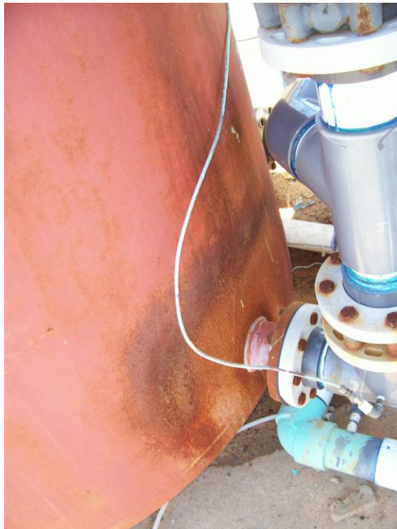
Severe corrosion on filter tank
