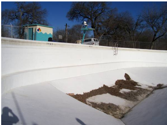
Slope along back wall of deep end violates 3:1 current Texas Department of State Health Services regulations.
