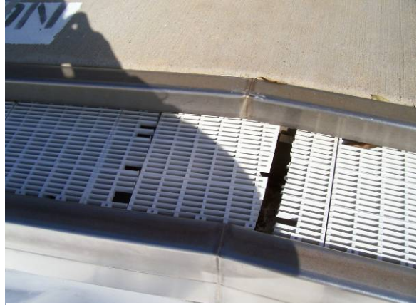
Broken PVC gutter grating
