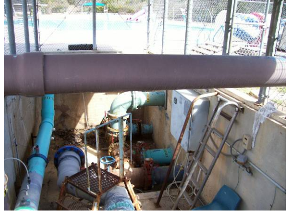
Pump pit is enclosed by a lockable chain link fence and covered by a roof.
