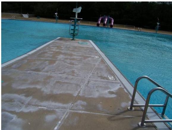
Chemical staining on deck.
