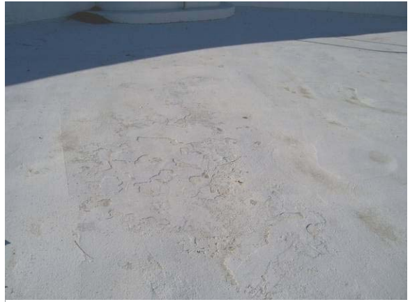
Rough condition of deck.
