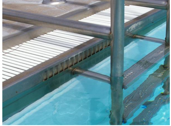
Surge weirs are not operating properly.
