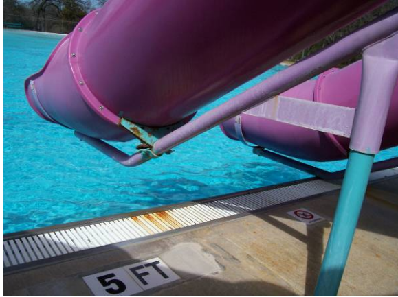
Corrosion on water slide equipment causing staining on gutter system.
