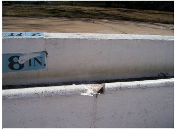
Broken gutter lip.
