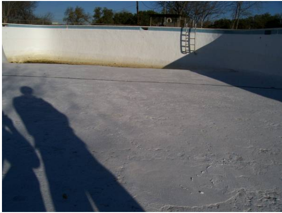
Rough condition of pool deck.
