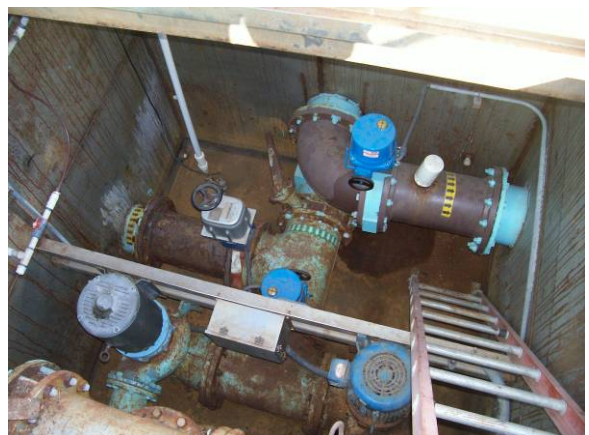
Corrosion of objects inside pump pit.
