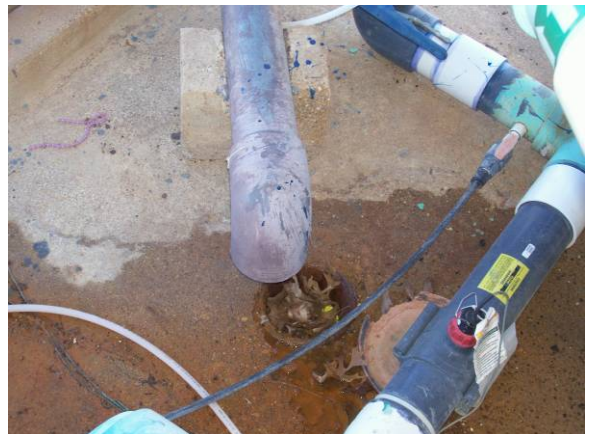
Misalignment of backwash line and sanitary sewer drain causes mechanical area to flood.
