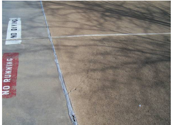
Hair line crack, failing expansion joints
