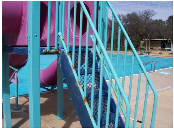
Corrosion on the water slide platform.
