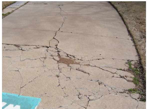
Outer sidewalk shows severe cracking.
