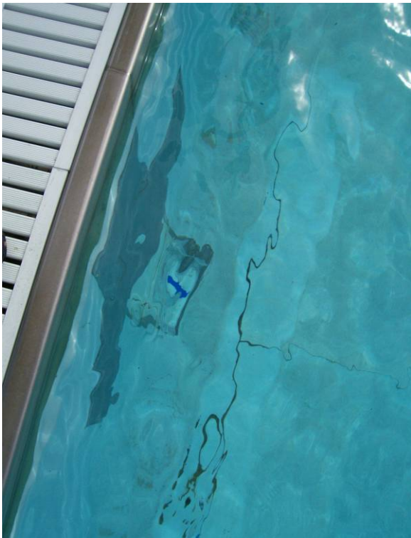
Large tear in PVC liner at wall target.
