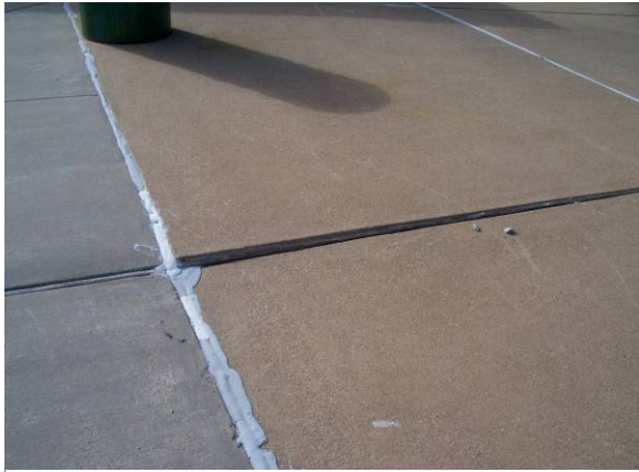
One slab has lifted slightly.
