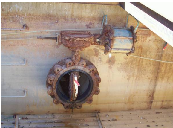
Automatic valves are in poor condition. Replacement parts are no longer manufactured.
