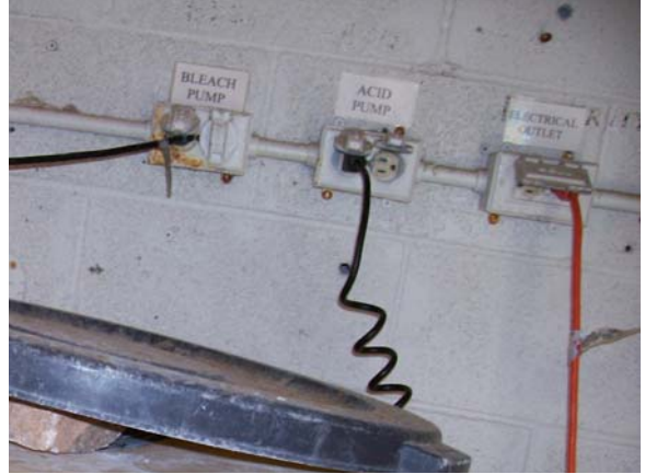
Electrical outlets without GFI protection.
