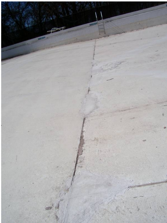
Multiple patches and rough condition of pool shell.
