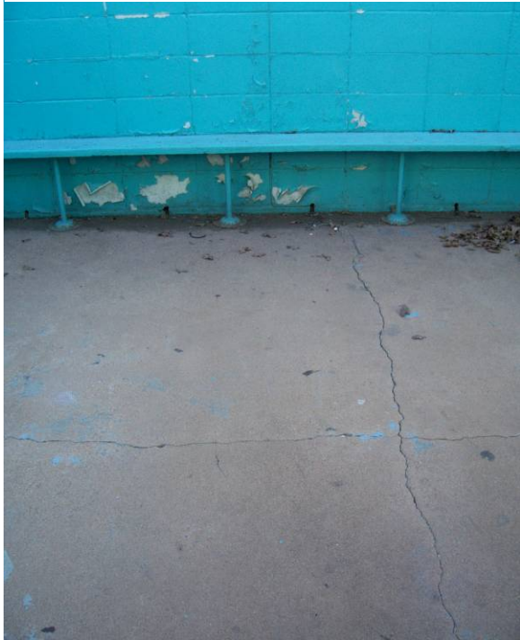
Cracked floor and failing paint in bathhouse. (Reported to be repaired during annual maintenance for 2007 season.)
