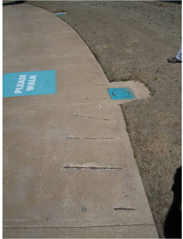
Exposed rebar in pool deck.
