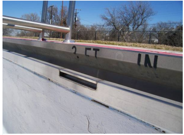
Overflow weir, failing caulk seal along gutter, poor condition of vertical depth markers
