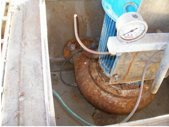
Severe corrosion on recirculation pump
